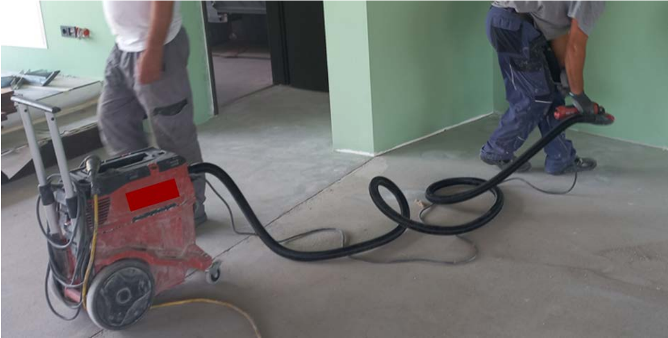
The worker on the right also uses a hand-held tool with on-tool dust control, on the left one can see the industrial dust extractor ensuring dust extraction.
